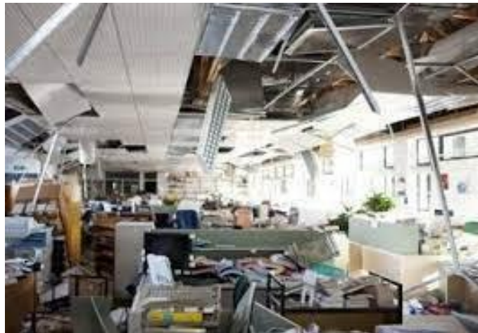
FIGURE 15: COLLAPSE OF FALSE CEILING
