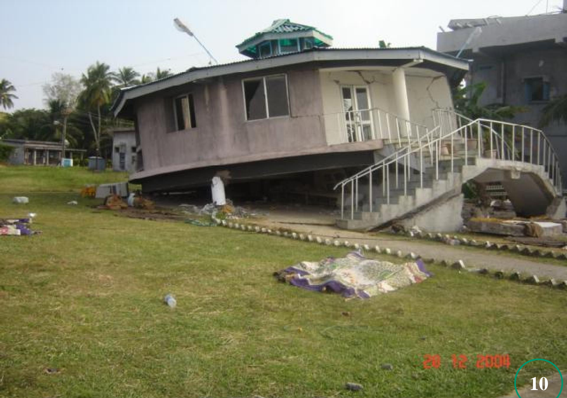
DAMAGED ATC - ANOTHER VIEW
