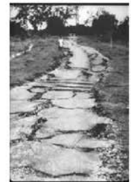
Cracks in upper Assam Trunk Road
