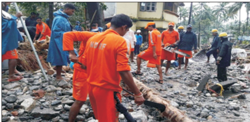
Figure 7.3 : NDRF personnel clearing debris after landslides and floods
