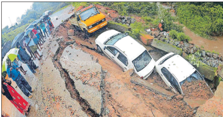
Figure 4.7 : Destruction of Roads
