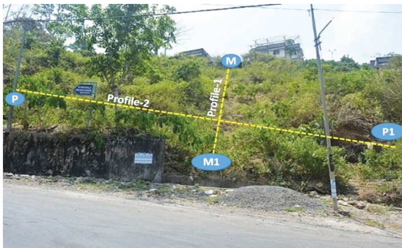
Figure 4 : Kamaraj Landslide at Brookshabad, Port Blair
