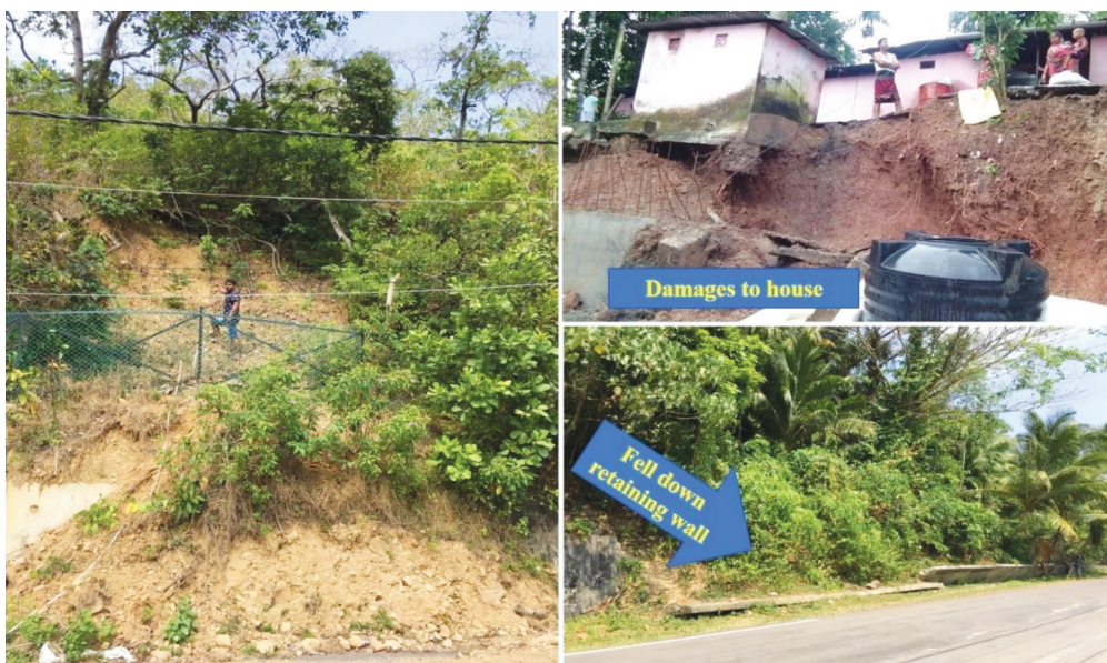
Figure 8 : Landslide Damage in some other Sites of Brookshabad, Port Blair after Cyclone ‘Vardha’
