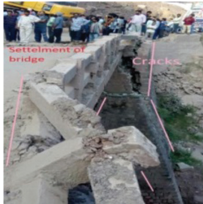
Photo 4: Settlement of bridge and Cracks in bridge abutment A2.
