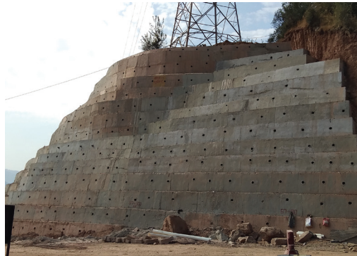
Photo 16: High Tension Tower Ch 87 + 886 km
