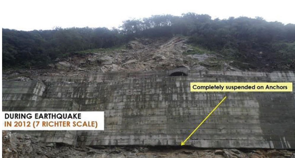
Fig. 5.17: Condition of stabilised slope with prestressed cable anchor after 2012, earthquake (Magnitude 7)
