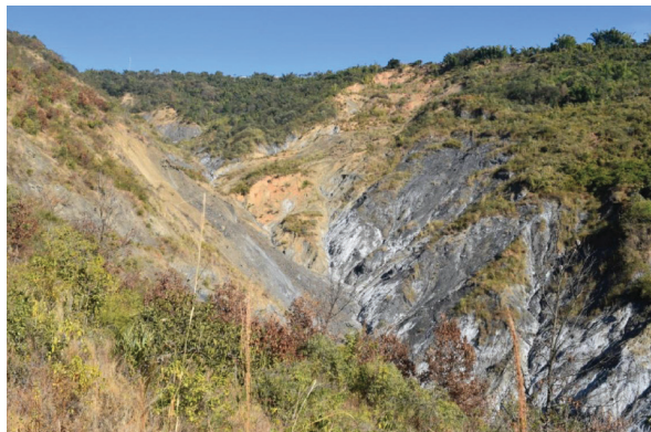
Fig. 7: View of the slide affected area
