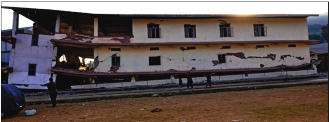
Figure 25: - Collapse of first storey of building at Saikul bazaar in sadar hills due to soft storey.
