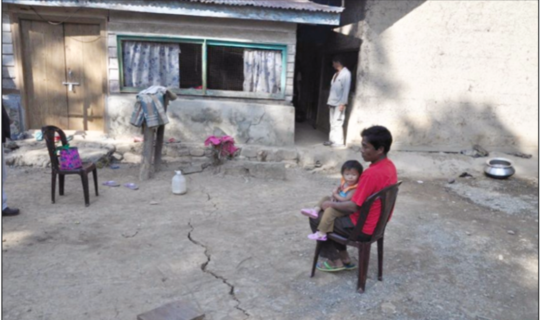
Figure 35: - Cracks observed in a masonry building with cement mortar bond at Leimakhongarea Manipur.
