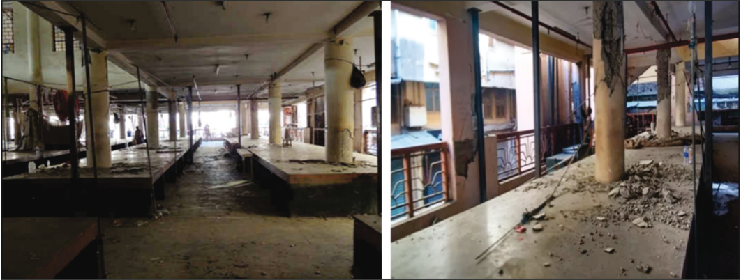
Figure 18: - Damaged Imphal Ima Market
