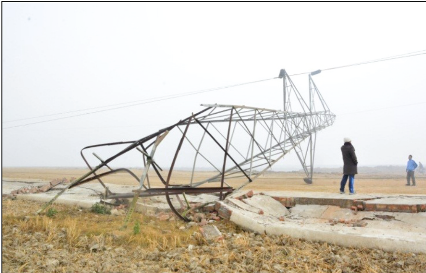
Figure 17: - Failure of power line near Noney.
