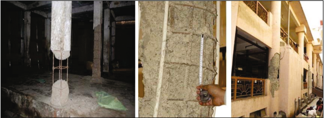
Figure 30: - Base of first storey column with widely spaced ties and spalled concrete, (Bishnupur Market.) and new market
