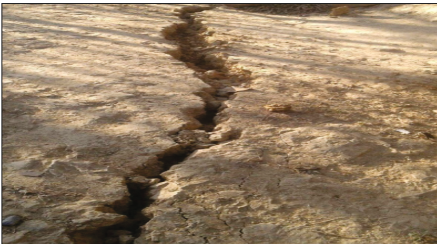
Figure 15: - Showing major cracks developed in Kabui Khullen village in Tamenglong district
