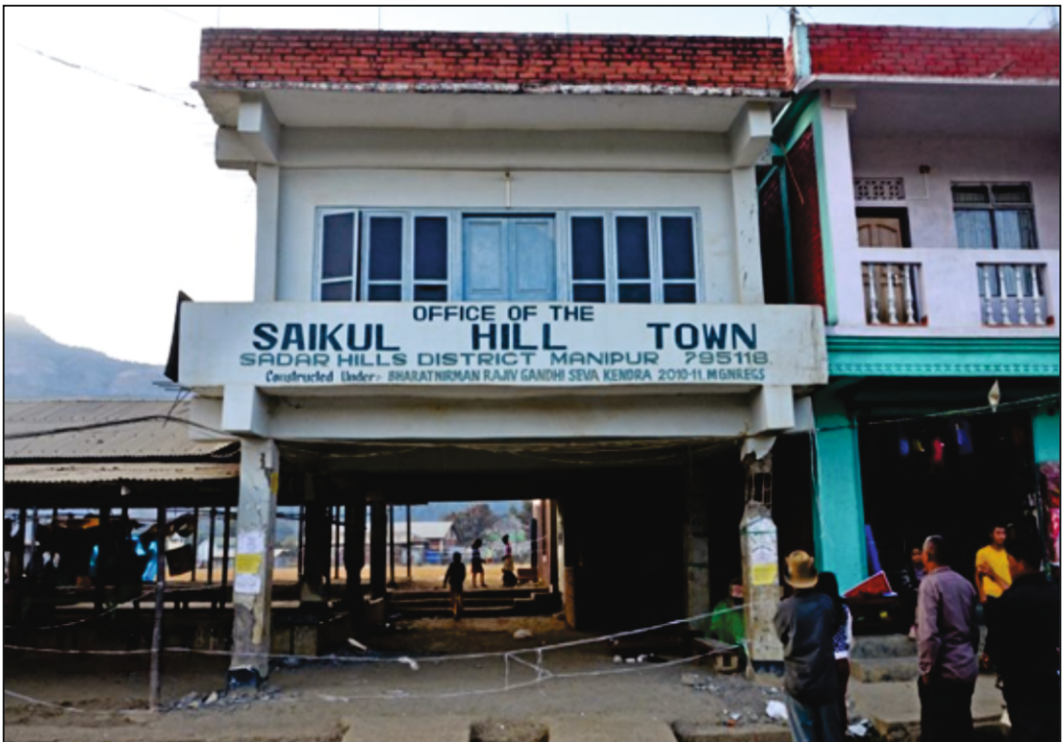
Figure 27: - Failure of columns due to soft storey in Saikul bazar, Sadar hills.
