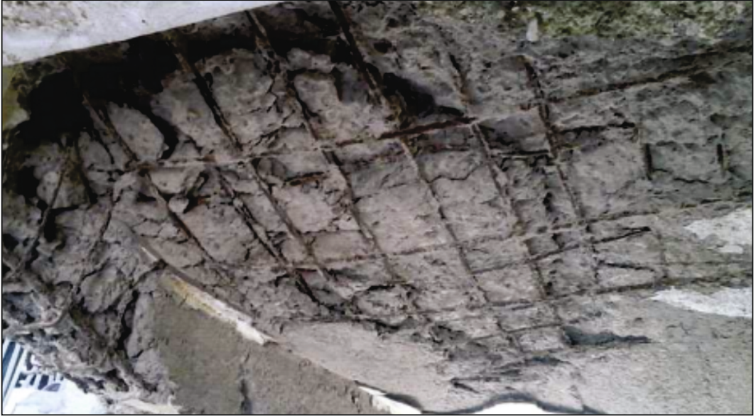
Figure 29: - Corroded reinforcement in slab, beam at Government Polytechnic building, Manipur.
