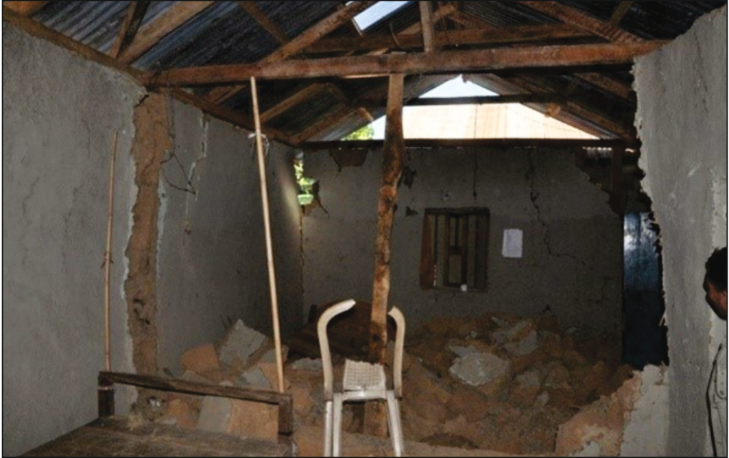
Figure 36: - Collapsed Mud wall house near the epicenter region Noney, Tamenglong.
