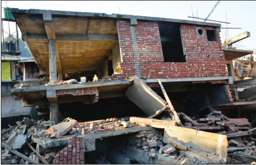
Figure 16: - Collapse of a two-storey building in Keishampat, Imphal.
