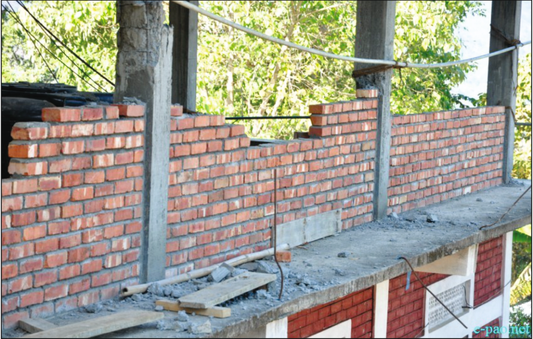
Figure 23: - Short column effect due to presence of partial infill walls at Tamenglong, Manipur.
