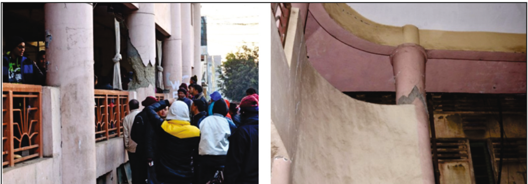
Figure 24: - Column damages due to short column effect in Imphal.
