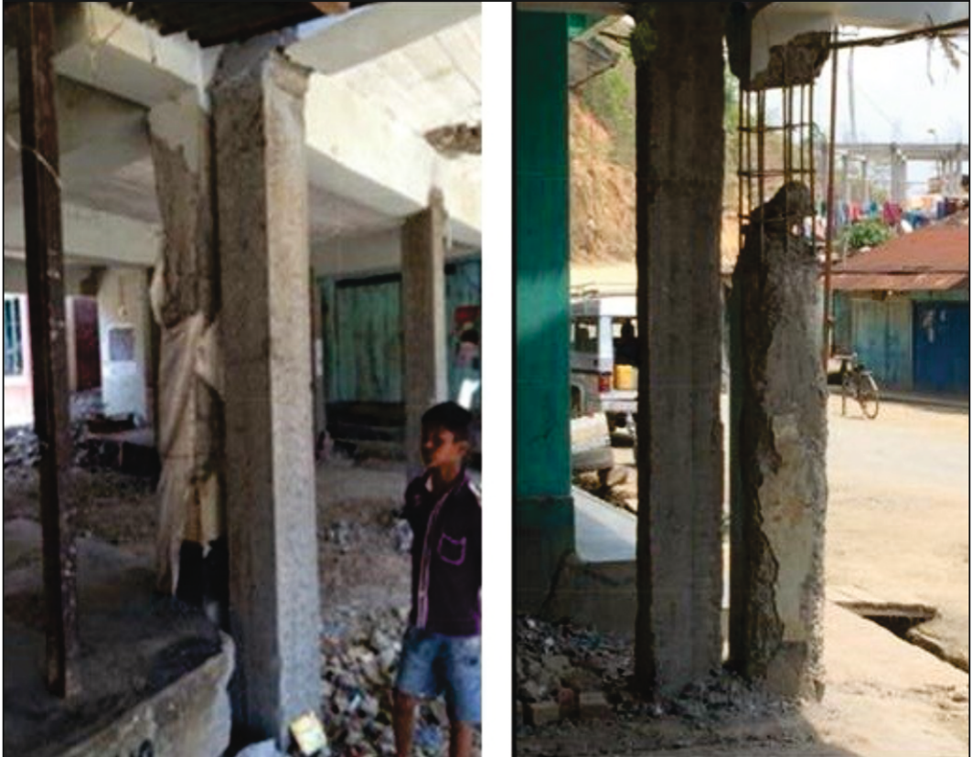
Figure 47: - Propping damaged RCC structures by newly constructed columns not connected to the beam above in Saikul.
