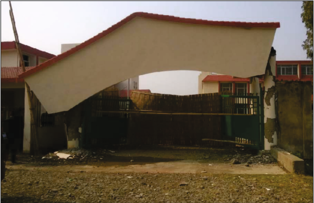
Figure 33: - Damaged Central Agricultural University gate due to landfill soil.
