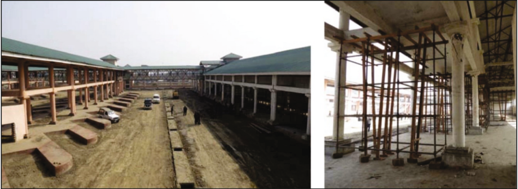
Figure 45 : - Severe damage to RC columns at the Inter-State Bus Terminal, Imphal after the earthquake
