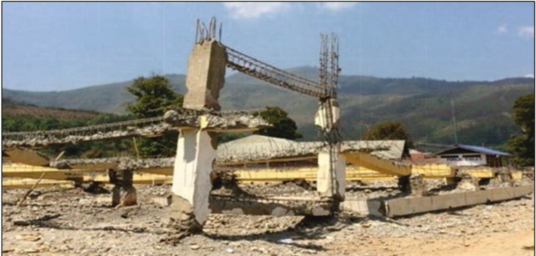
Figure 32: - Collapsed frame of a soft-storeyed RCC structure (women vendor's market) in Saikul.
