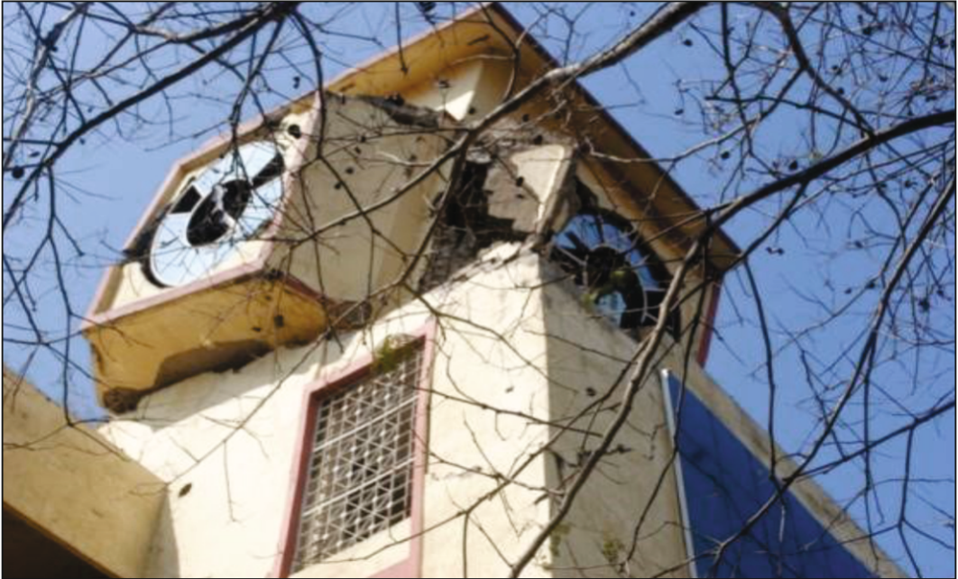
Figure 28: - Damaged building due to mass irregularity at Govt. Polytechnic, Takyelpat.
