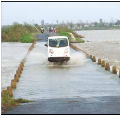
Figure 9: Damaged and flooded road
