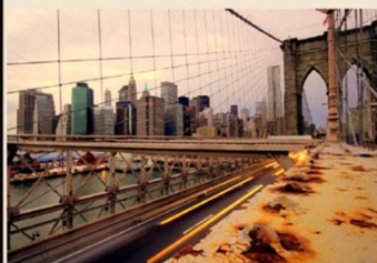
A view showing the corrosion of The Brooklyn Bridge, a National Historic Landmark, New York.
