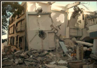
A view of collapsed Reinforced Concrete Building during Bhuj Earthquake, Gujarat.
