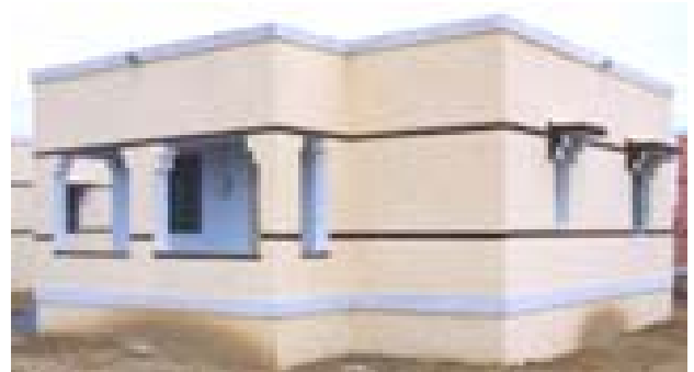
An earthquake resistant house of Seismic Zone V (MSK IX or more):- Single storeyed, one brick thick walls in 1:4 cement-sand mortar, with seismic bands at plinth, window sill and lintel level, as well vertical bars at all corners is shown as constructed in Gujarat after 2001 earthquake.
