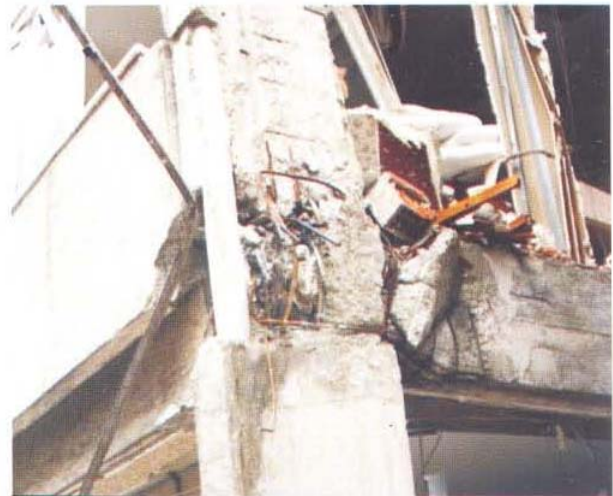
Fig.7:- Failure in column-beam joint (lack of stirrups)
