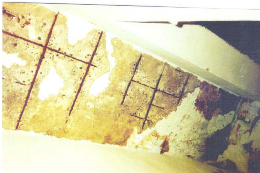
Fig.12:- Corrosion in the RC slab (lack of control on the cover)
