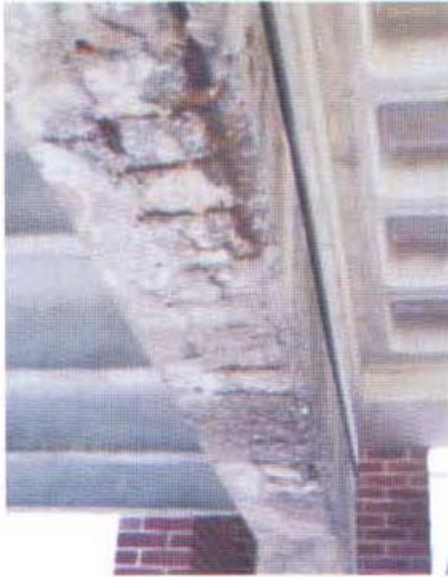
Fig.10:- Corrosion in RC beam
