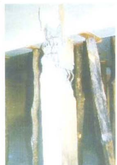
Fig.3:- Cracks in column
