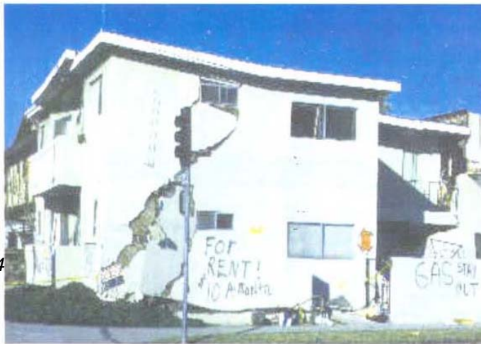
Fig.4:- Cracks in masonry wall
