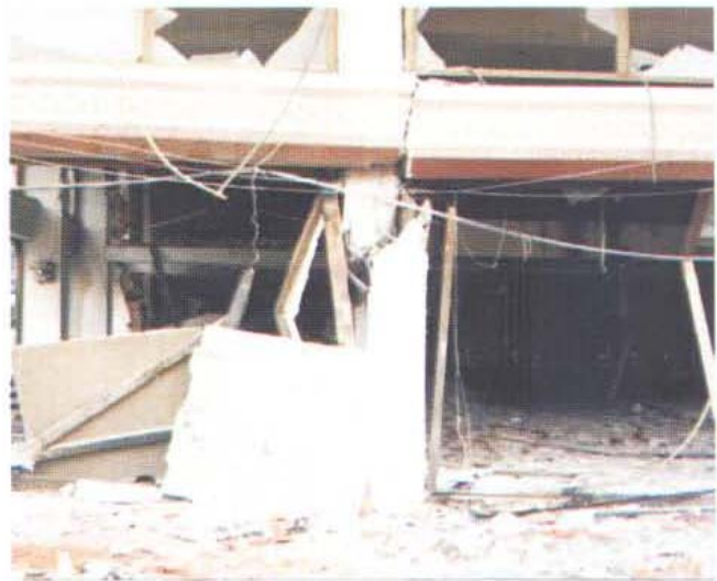
Fig.9:- Column top failure (bad joint detail)
