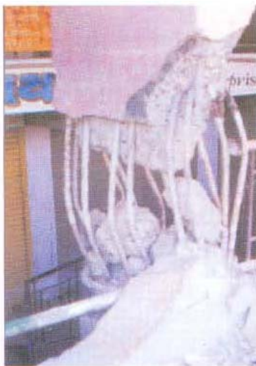
Fig.8:- Column failure (absence of tiers, buckling of longitudinal bars)
