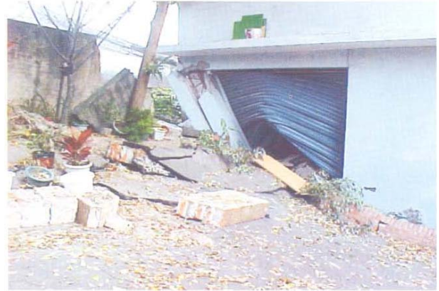
Fig.13:- Damage of building due to ground failure
