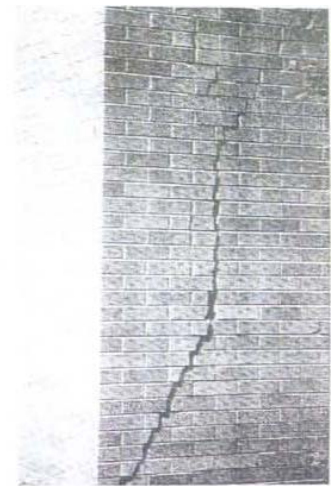
Fig.5:- Cracks in good quality brick wall
