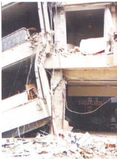
Fig.6:- Failure of a portion of building (at expansion joint)
