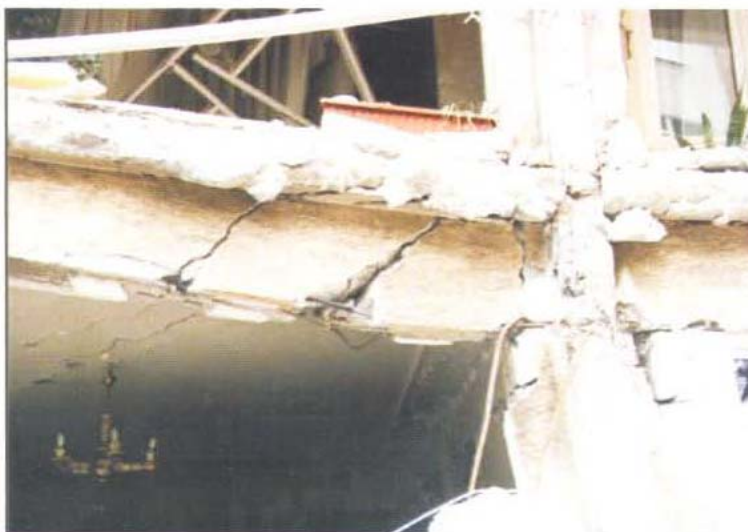
Fig.2:- Diagonal cracks of the beam and failure at the column top
