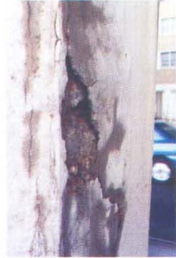
Fig.11:- Corrosion in the RC Column
