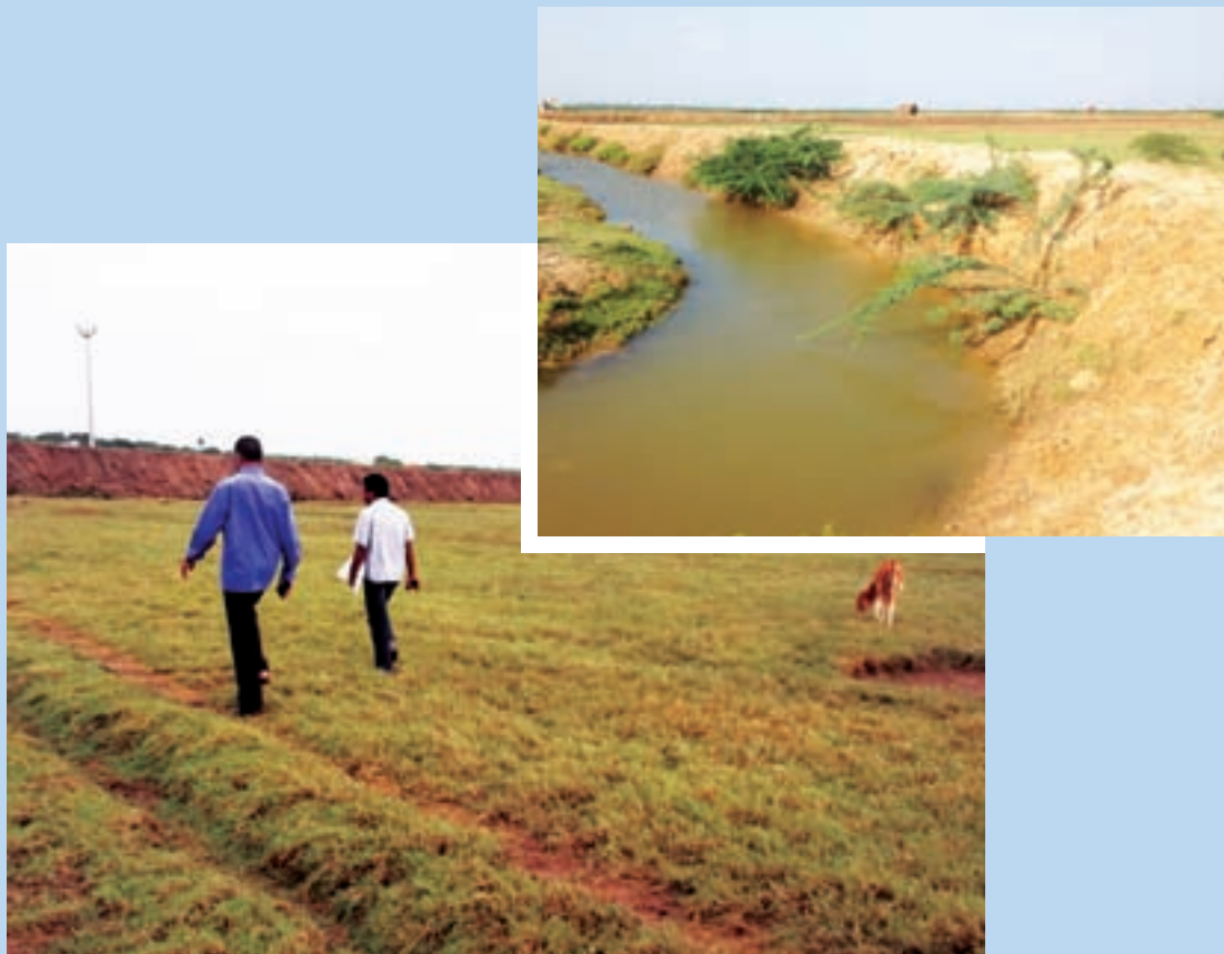
Pic 3: Bund Strengthening and Shutter Construction at Kumarakudi, Nagapattinam District, Tamil Nadu
