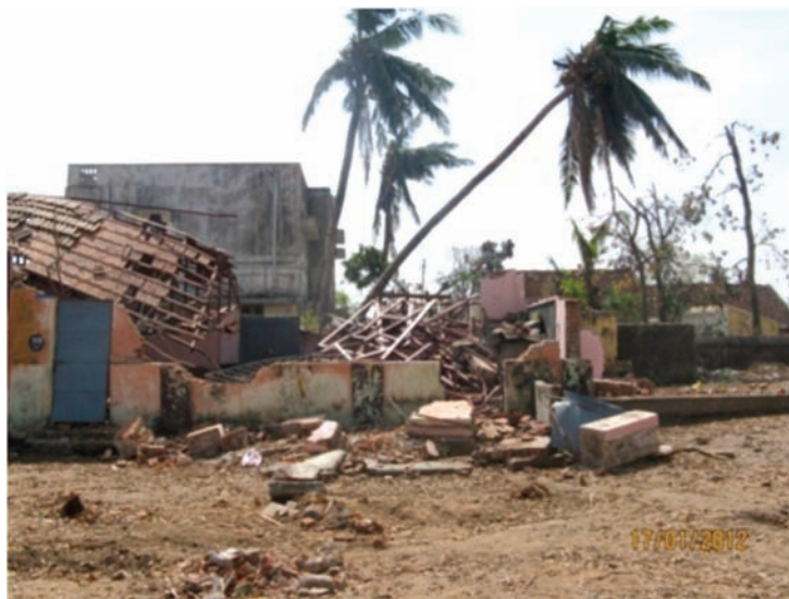
A school damaged in Cuddalore
