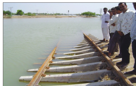
Damage caused by the floods
