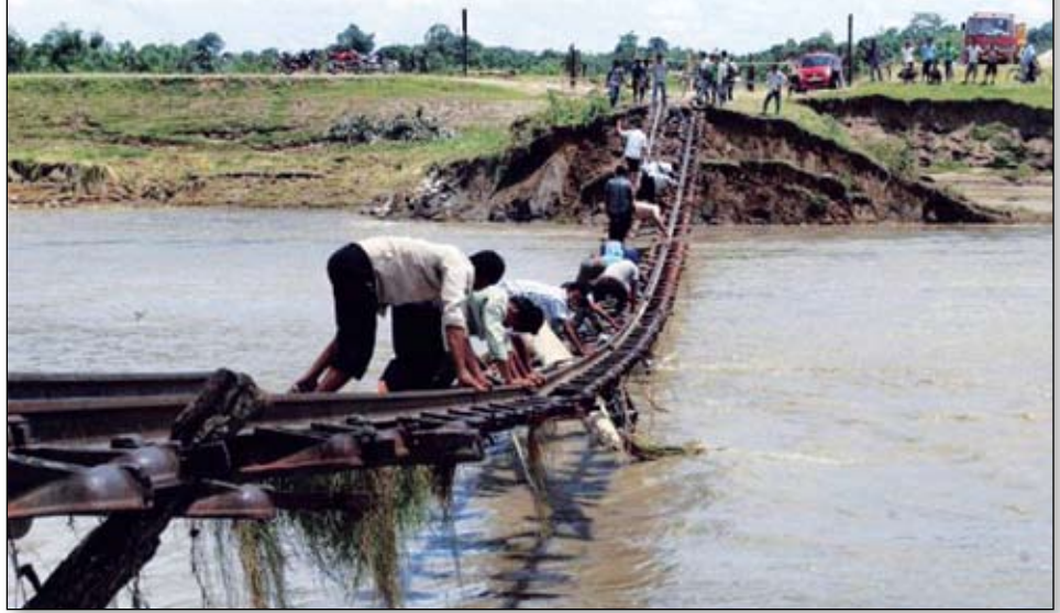
PERILOUS CROSSING: People make use of a wrecked railway track to negotiate the flood waters at Tokobari, in Dhemaji district of Assam. Photo: www.thehindu.com, 19 Aug 2011.
