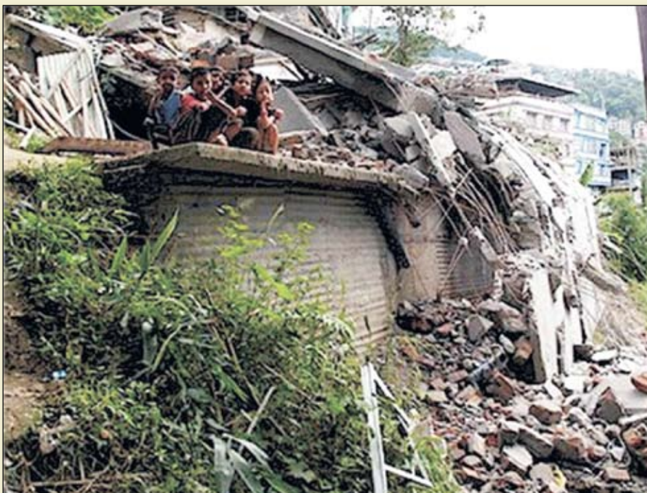
Damaged School building in Sikkim (Photo: Seedsindia)
