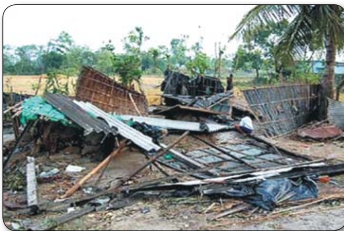
Picture showing damages houses in Jaipauri, West Bengal
