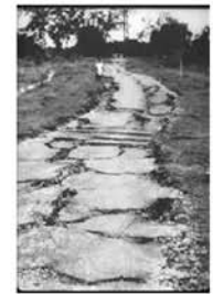
Cracks in upper Assam Trunk Road
