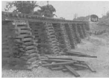
Subsidence of railway embankment replaced by wooden sleepers in Dum Duma
