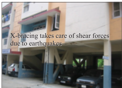
Soft storey at the ground
