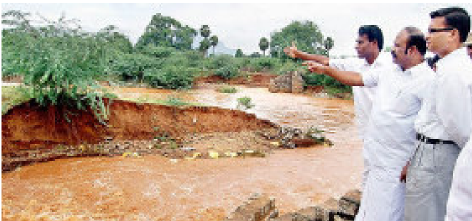
Assessment: Minister for Hindu Religious and Charitable Endowment K.R. Perikaruppan, middle, and Sivaganga Collector Pankaj Kumar Bansal, right, inspecting a damaged causeway near Singampunari on Thursday.
